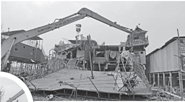
Following a The Daily Star report, the officials took steps to demolish the illegal structures on the Meghna riverbanks.
