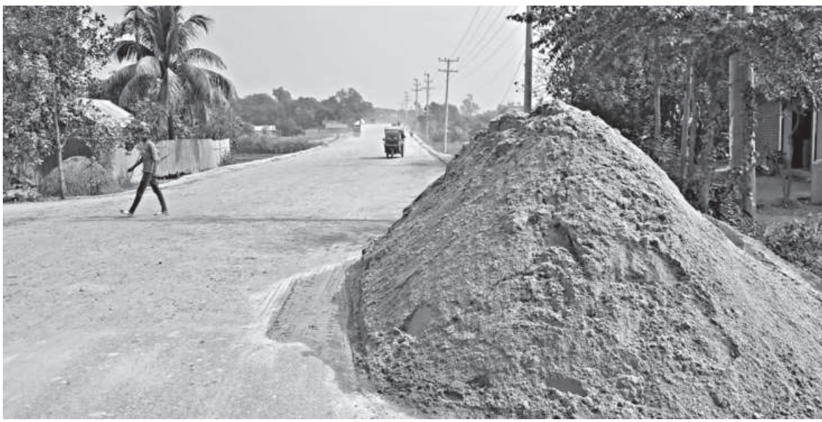
Even though the contractor withdrew the entire Tk 53 crore bill for the construction work of Nabinagar-Shibpur-Radhika regional highway in Brahmanbaria, the road remains incomplete.
