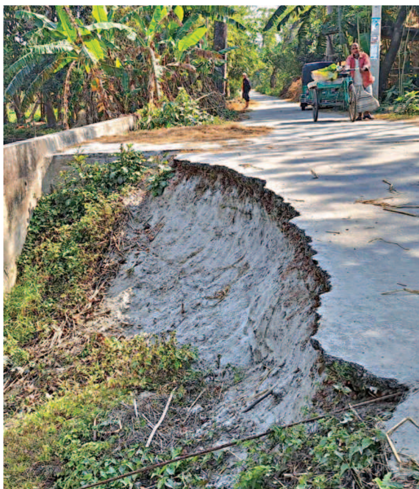
A portion of a road in Aicha village of Barishal's Sadar upazila caved in due to heavy downpour almost three years ago. While the authorities concerned continue to turn a blind eye, locals keep suffering. The photo was taken yesterday.
