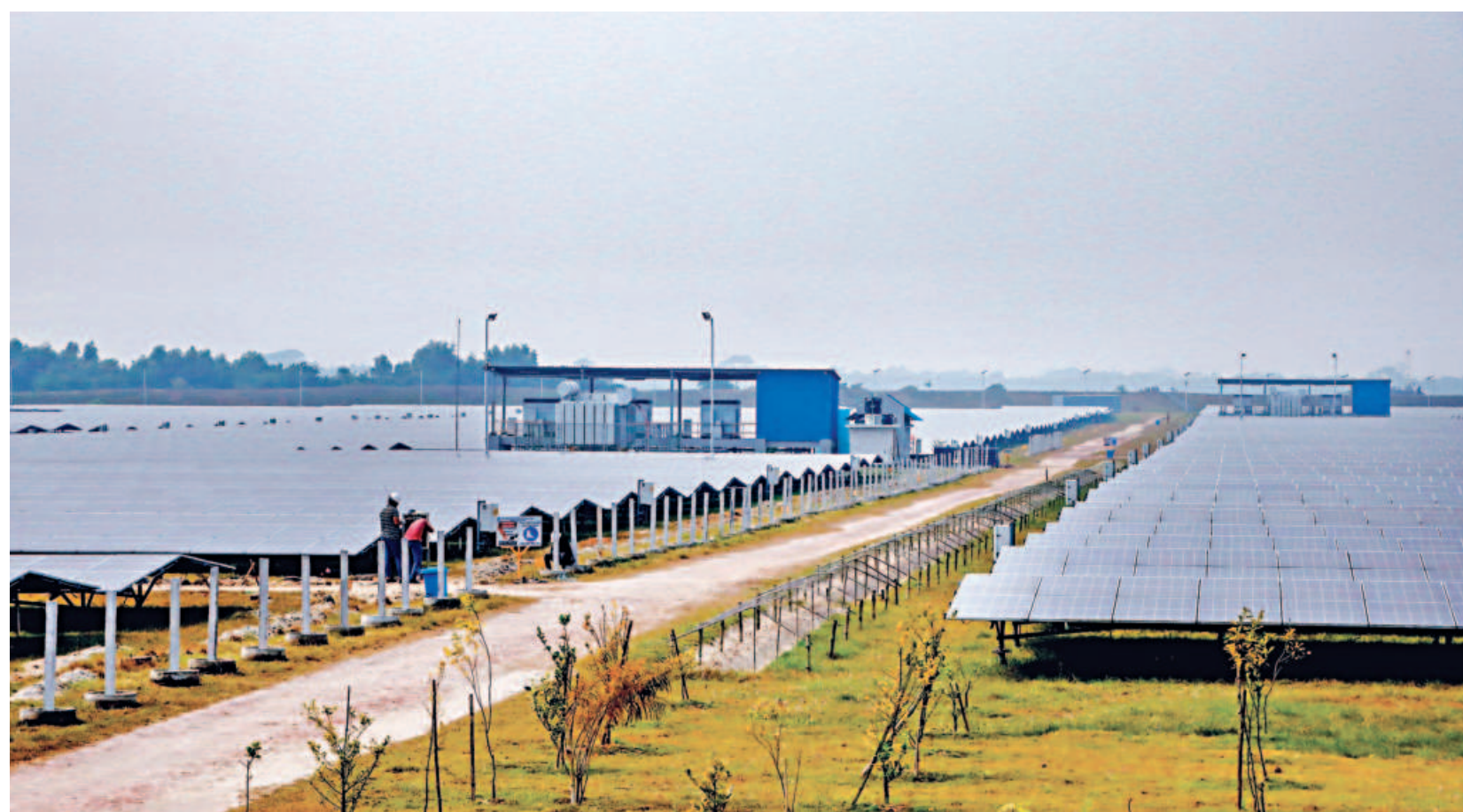
The 100MW Energoan Solar Power Plant at Borodurgapur in Mongla, Bagerhat.
