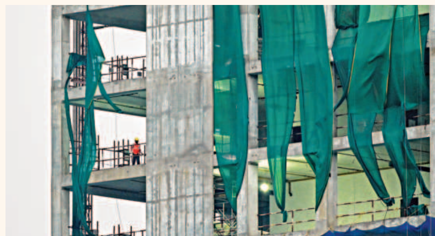
A labourer works at the construction site of a new high rise building in Mumbai. Much of Prime Minister Narendra Modi's government spending in recent years has gone into building infrastructure, while private investment and job creation have lagged.
