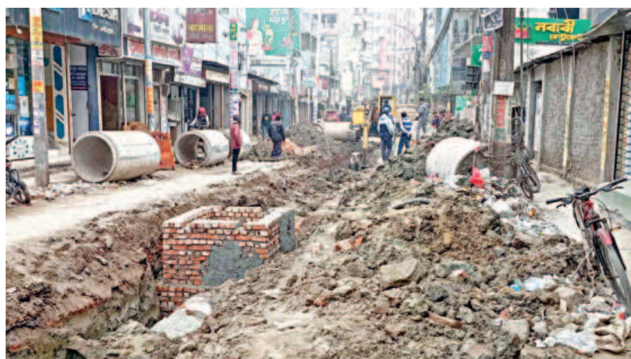
People struggle to cross the Saheb Ali Road as the street has been dug up for drainage development work, leaving it almost unusable.
