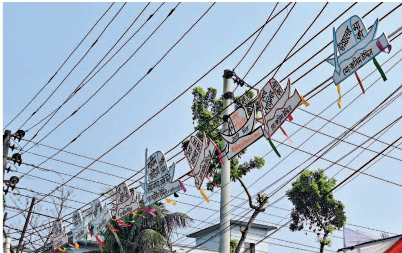
Campaign materials hanging from electricity cables are posing risk to road users in Barishal city's Amtala Mor area yesterday, nearly two weeks after the national polls.
