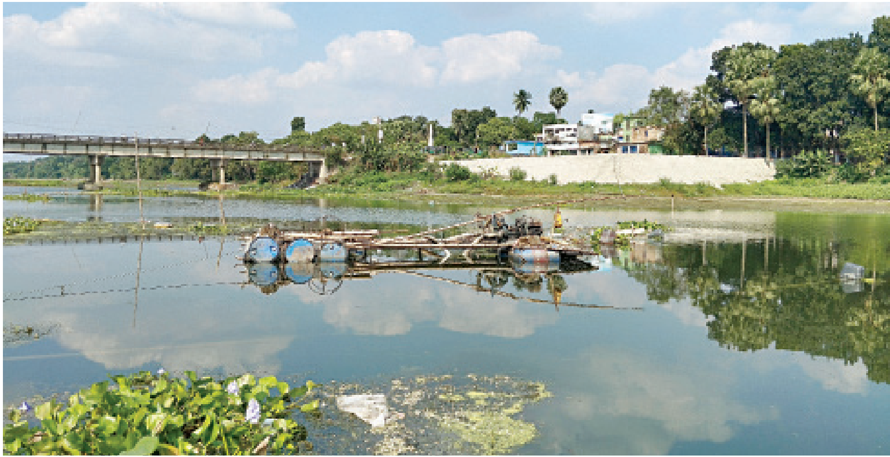
Sand being pumped to the shore via large pipes to fill up the bank of the Kumar river, inset, to construct a bus stand in Magura's Sreepur upazila. The photo was taken recently.
