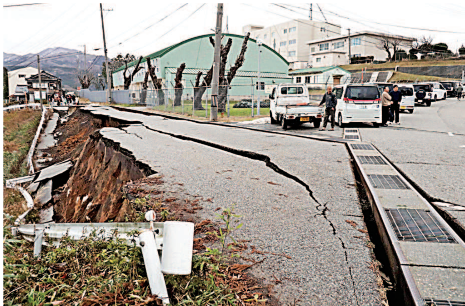
People stand next to large cracks on a road in the city of Wajima after a major 7.5 magnitude earthquake struck the Noto region in Ishikawa prefecture in Japan yesterday.
