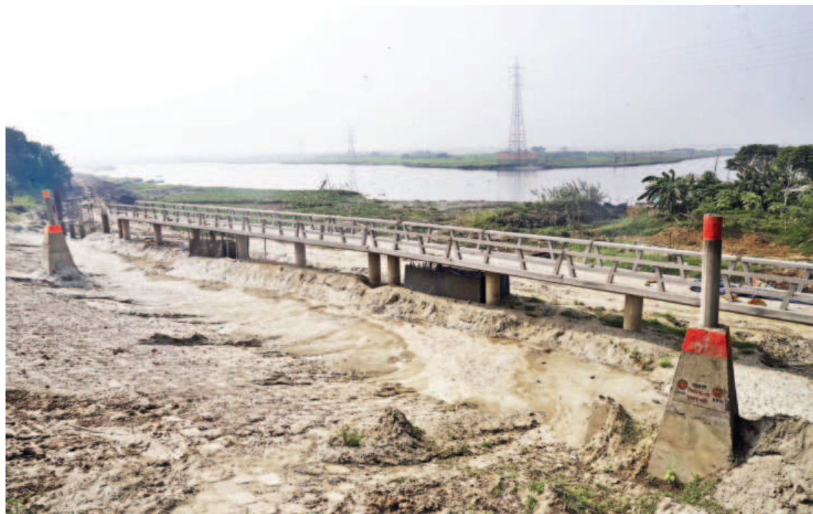
The BIWTA is building a walkway inside the area demarcated as the Turag river, violating a 2009 High Court directive on saving the rivers around the capital from encroachment. The photo was taken from Goran Chatbari near Mirpur Baribanh recently.
