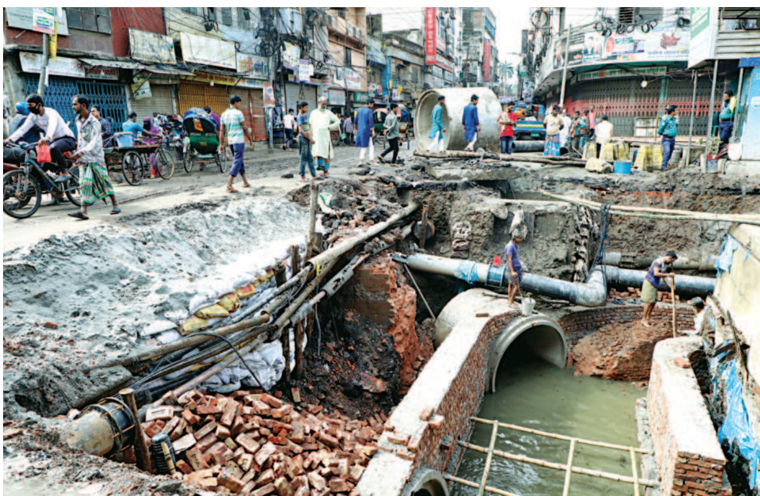
The drainage work on Midford road in Old Dhaka has been continuing for over a month without any protective measures. As a result, pedestrians and vehicles, mostly rickshaws and motorbikes, are forced to use the muddy road amid risk. The photo was taken yesterday afternoon.
