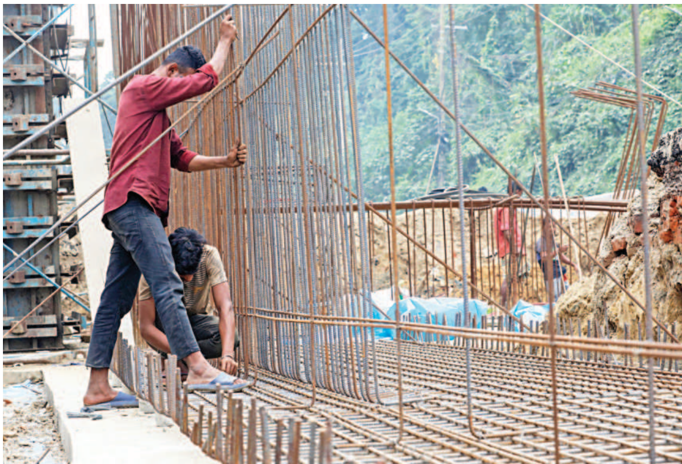
Workers are seen laying MS rods at a construction site in Chattogram city yesterday. Demand for the key construction material has been in a tailspin ever since the BNP and its allies started calling nationwide blockades and strikes, which are hampering development works.
