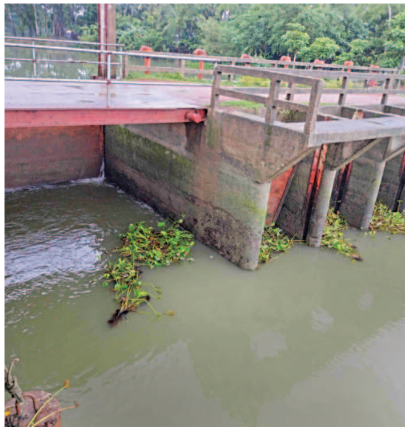
Lack of maintenance and operator has rendered this sluice gate on Panguchi canal in Morrelganj upazila useless.
