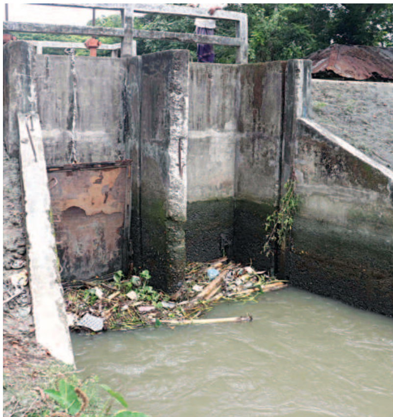
The sluice gate on Dadhibhanga canal in Pirojpur's Mathbaria upazila remains inoperative for lack of maintenance, blocking water flow.
