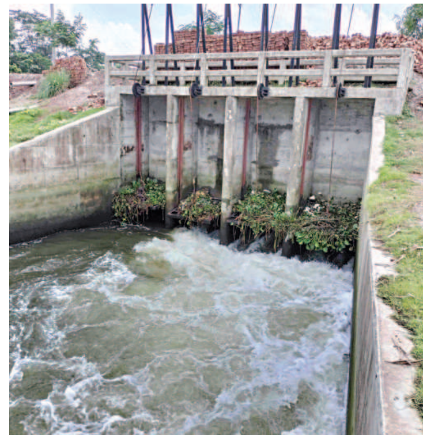
Due to the inactive sluice gate on Rayendra canal in Sarankhola upazila of Bagethat, water cannot flow smoothly.
