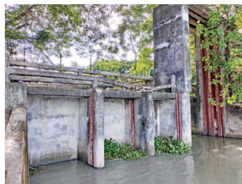
A damaged sluice gate on Kalakhali canal in Pirojpur Sadar Upazila.
