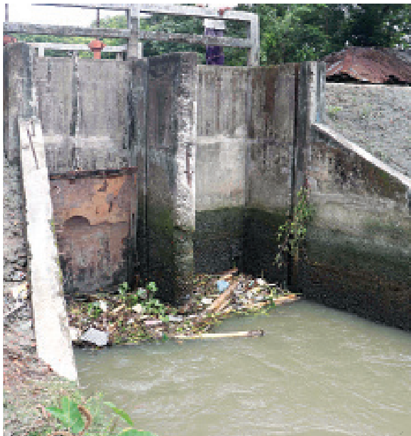
The sluice gate on Dadhibhanga canal in Pirojpur's Mathbaria upazila remains inoperative for lack of maintenance, blocking water flow.
