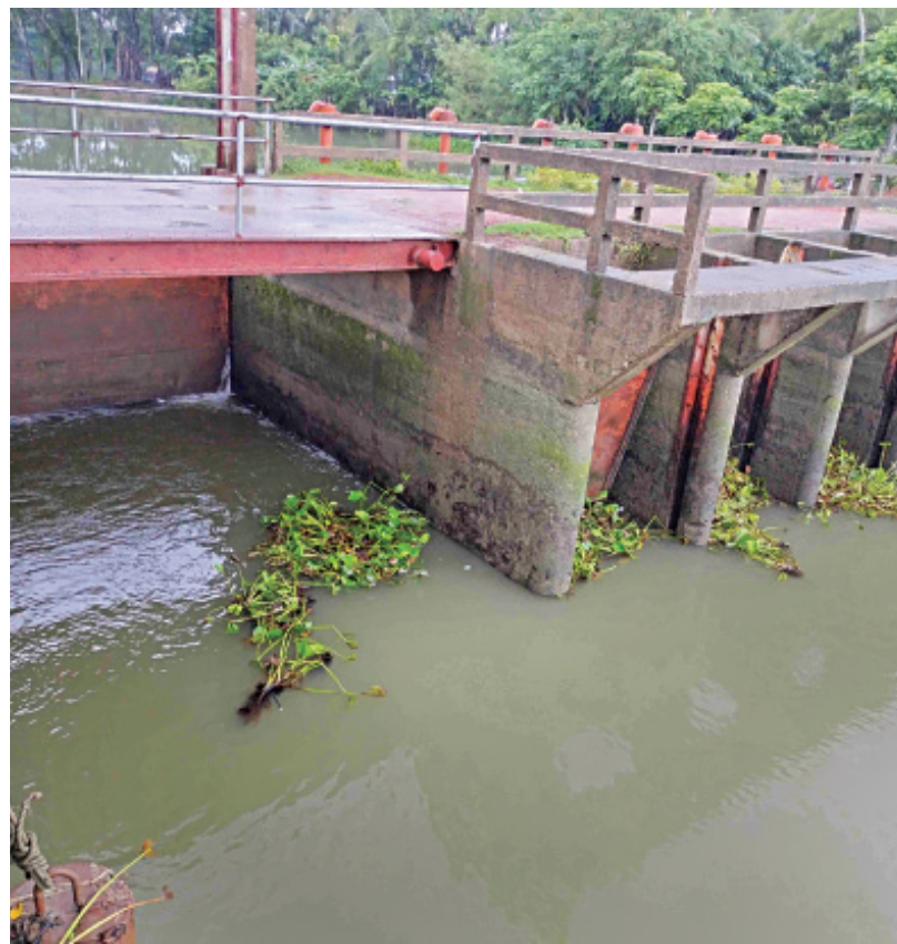
Lack of maintenance and operator has rendered this sluice gate on Panguchi canal in Morrelganj upazila useless.
