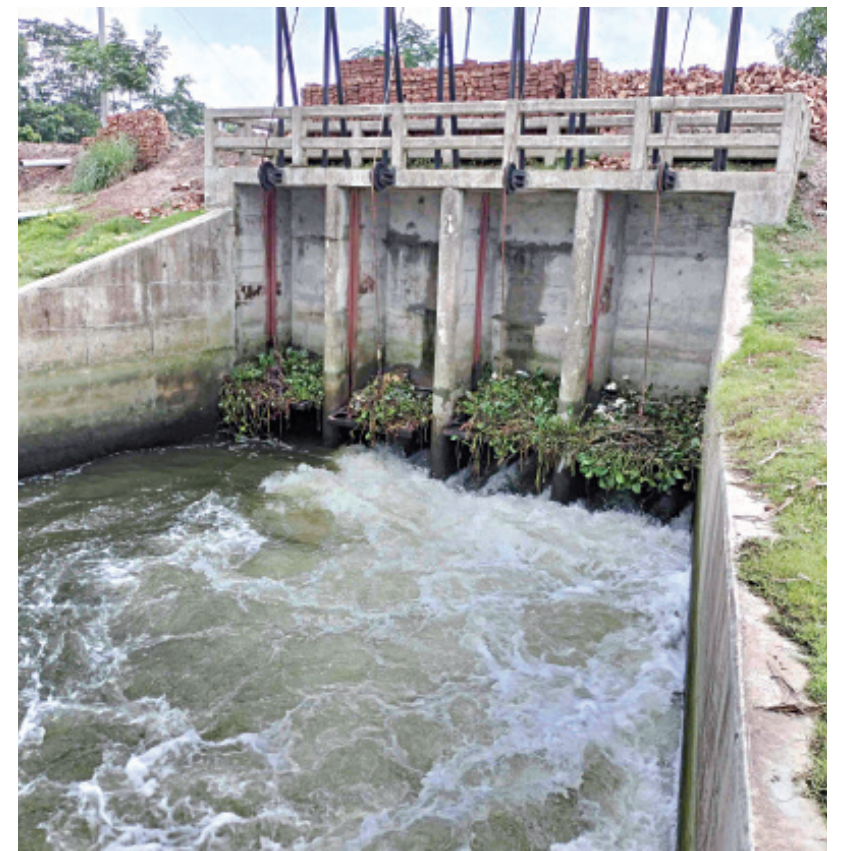
Due to the inactive sluice gate on Rayendra canal in Sarankhola upazila of Bagethat, water cannot flow smoothly.
