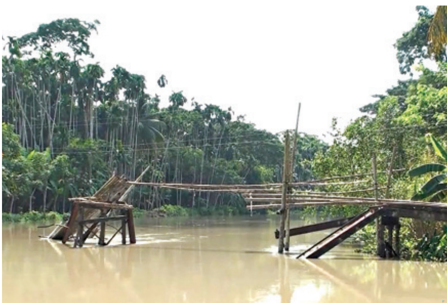
Constructed nearly two decades back, this iron-structured bridge over a canal in Bagerhat's Morrelganj upazila collapsed about four years ago. PHOTO: COLLECTED
