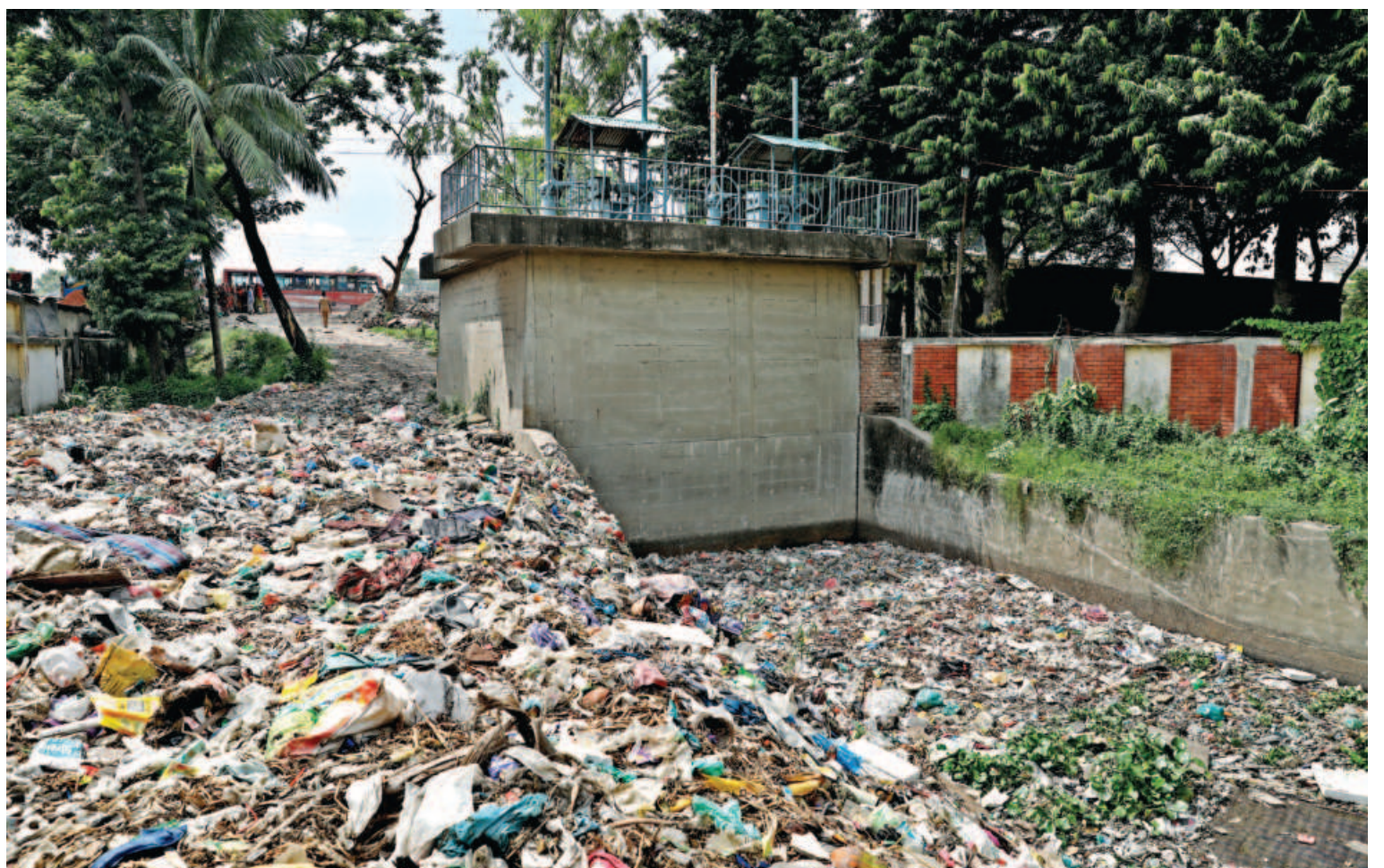
The pumping station for storm-water drainage in Kalyanpur is in a deplorable condition. Due to lack of maintenance by the authorities concerned, waste remains piled up surrounding it, resulting in constant waterlogging in the area. The photo was taken recently.
