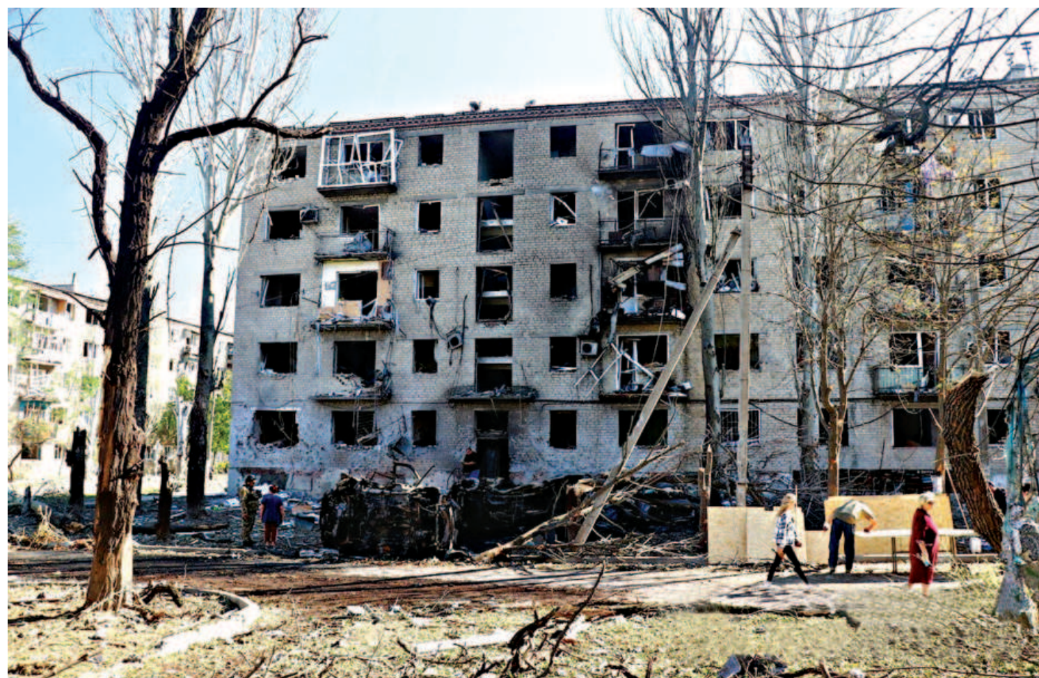
A view shows a destroyed residential building in the area damaged during a Russian missile strike in the town of Kurakhove, amid Russia's attack on Ukraine, in Donetsk region, Ukraine yesterday.
