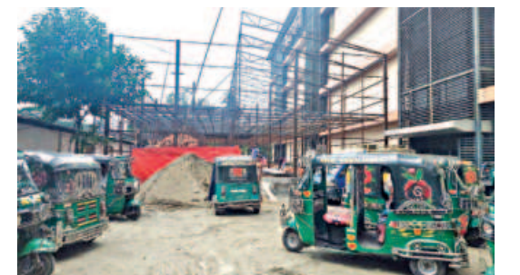
Work continues on this government land to illegally construct a building to "rehabilitate" hawkers in Noakhali. The photo was taken recently.
