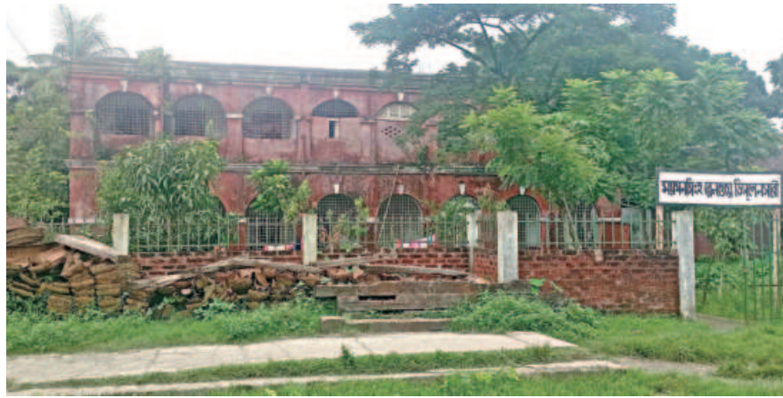
The Mymensingh railway dispensary is set up in a century-old building beside the station. The building is in a dilapidated condition and does not have necessary arrangements for patients.
