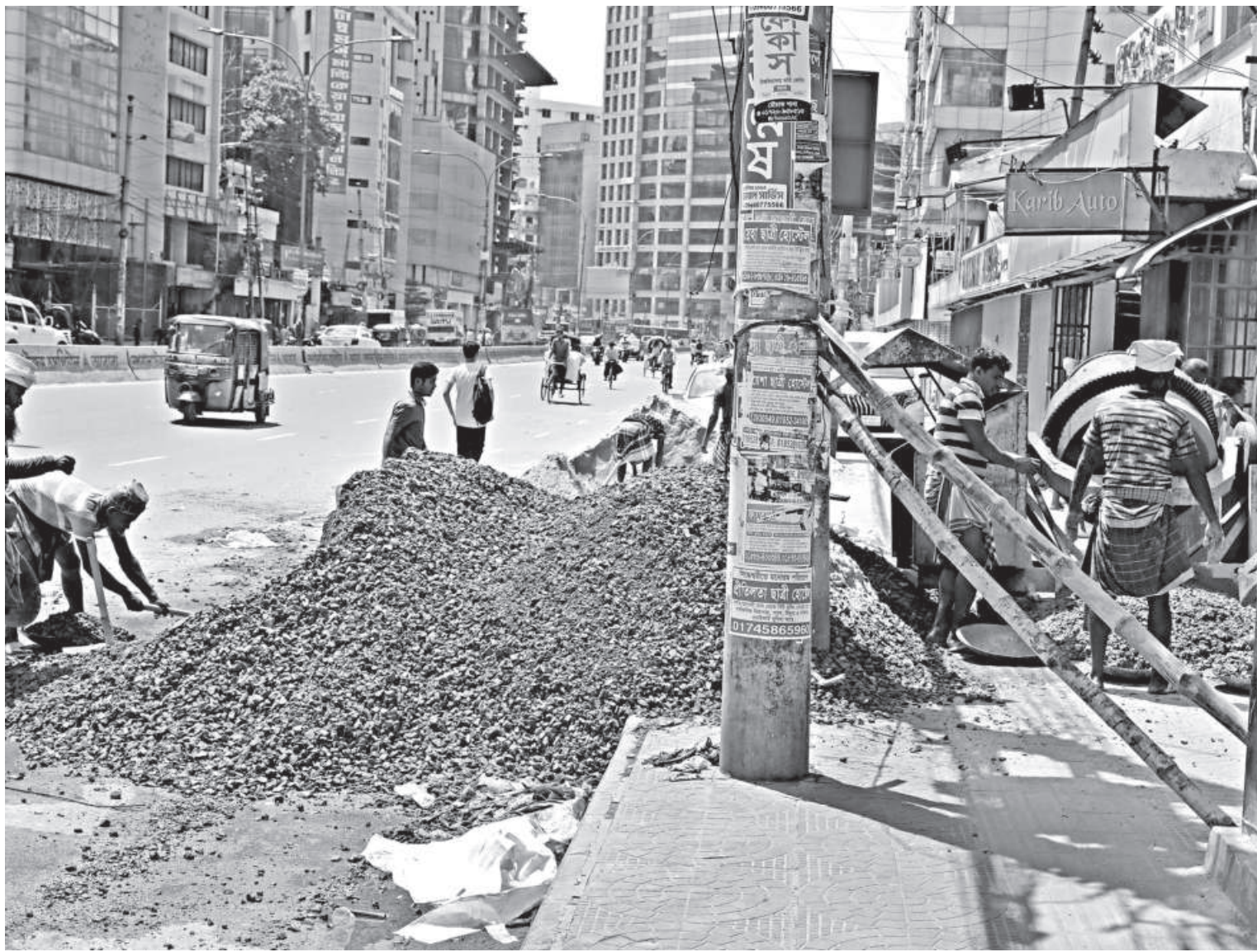
Construction work renders a portion of the road and most of the footpath unusable, causing problems for vehicles and pedestrians. Such a scene is common throughout the city almost all year round, with roads and footpaths being blocked off from public use. The photo was taken from the capital's Kakrail yesterday.
