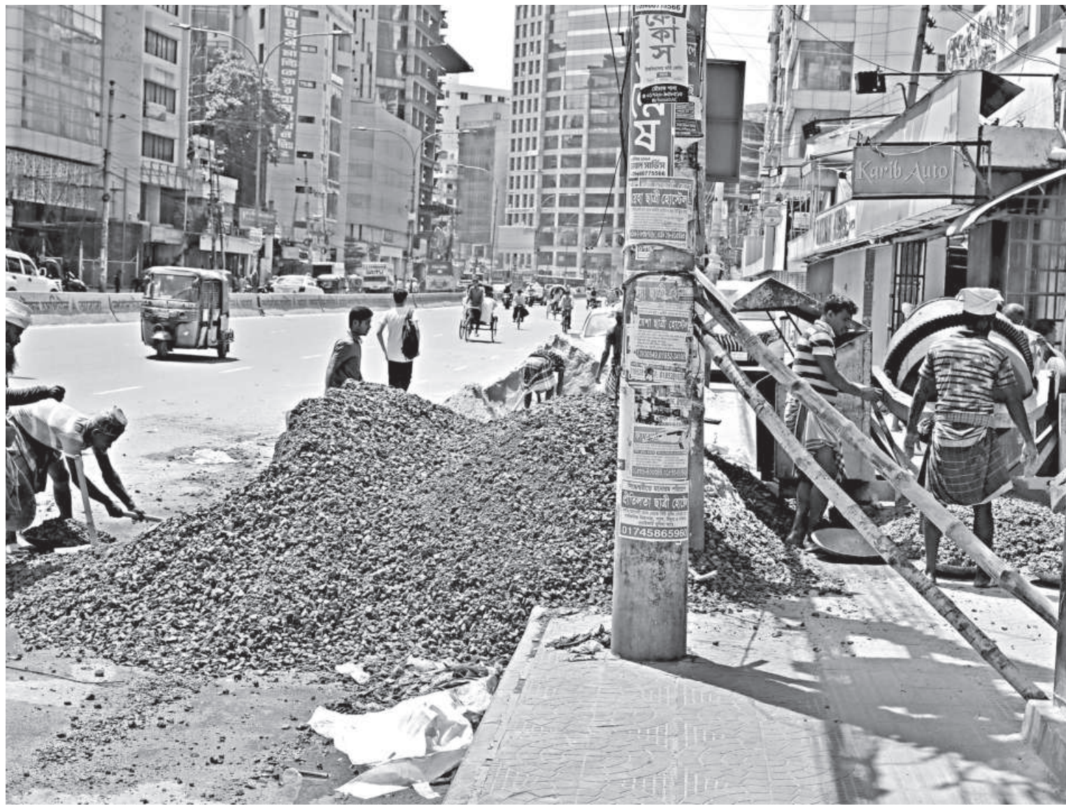
Construction work renders a portion of the road and most of the footpath unusable, causing problems for vehicles and pedestrians. Such a scene is common throughout the city almost all year round, with roads and footpaths being blocked off from public use. The photo was taken from the capital's Kakrail yesterday.
