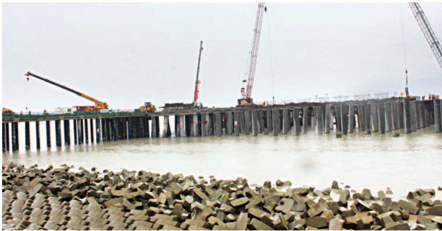
Work on the first terminal of the Payra Sea Port on the southern coast of Patuakhali is in full swing, with authorities hoping to begin operations by October. The completion of the terminal is expected to facilitate the transport of goods and speed up overall operations.
