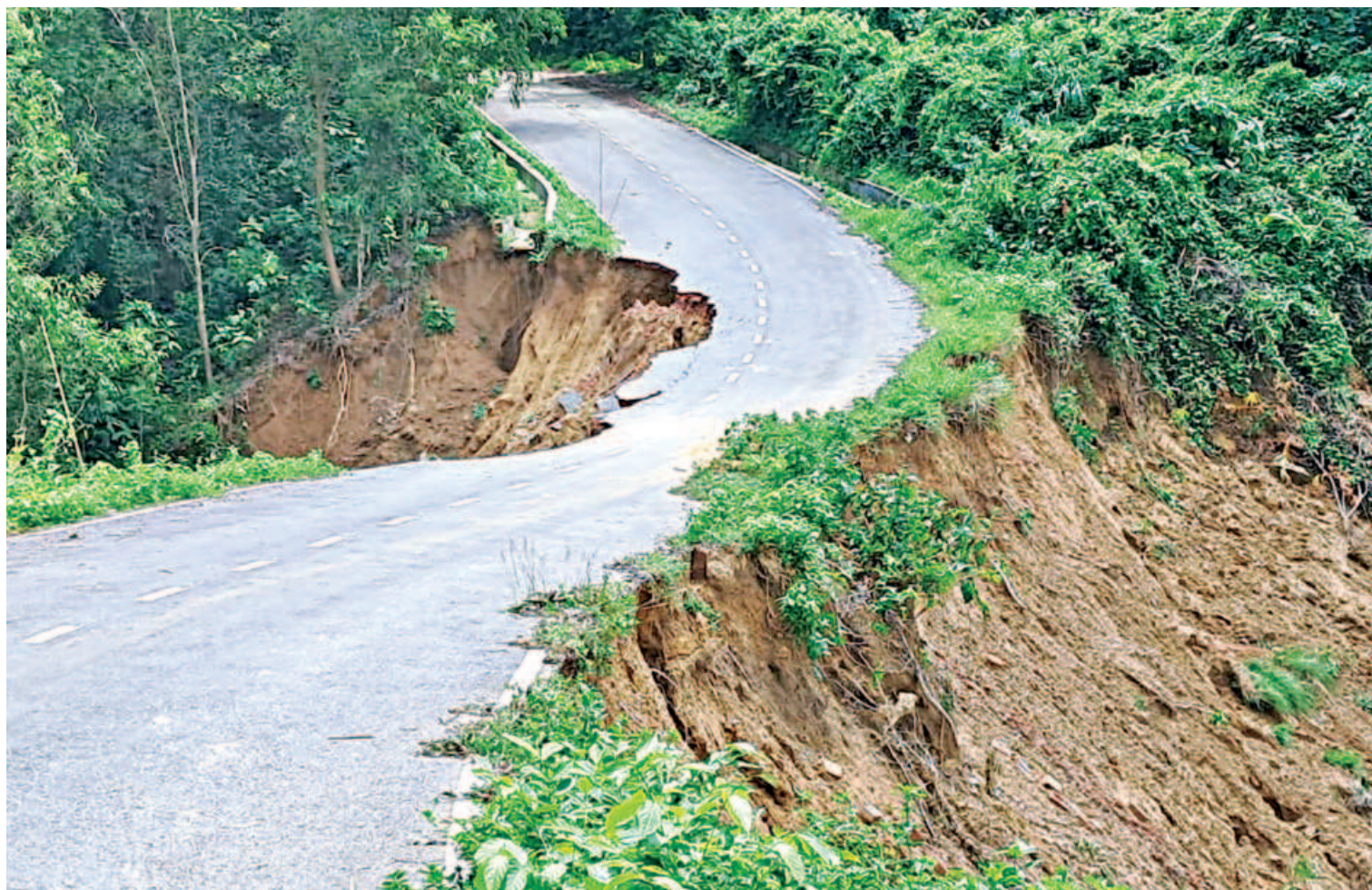
A portion of Bandarban's Lama Road has collapsed as heavy rains and severe floods caused extensive damages to the main roads and internal roads connecting various upazilas to the district headquarters. The photo was taken recently.
