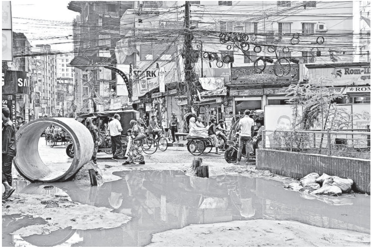
Dug around six months ago to deploy ring culverts to develop the area's sewerage networks, the Panditpara Road in Mymensingh city is yet to be repaired, leading to locals' woes. PHOTO: STAR
