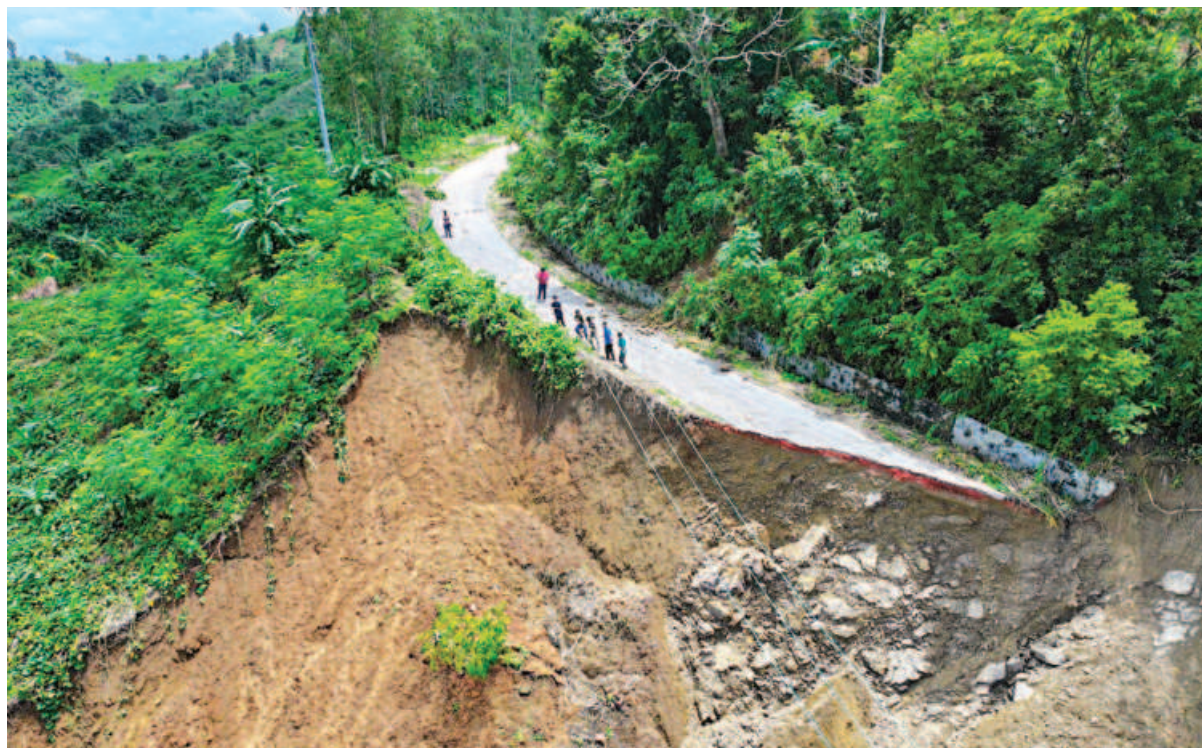
This part of Bandarban-Thanchi road collapsed after a recent landslide due to torrential rain. Workers of the power department have been working to restore electricity supply to the area. The road communications between Bandarban and Thanchi remains snapped. The photo was taken in Parilpar area of Thanchi on Friday.
