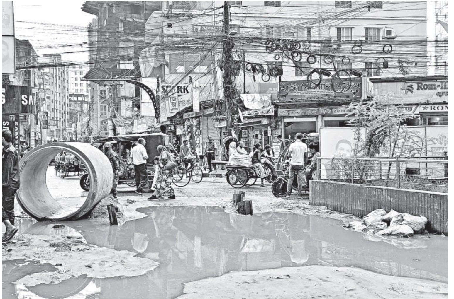
Dug around six months ago to deploy ring culverts to develop the area's sewerage networks, the Panditpara Road in Mymensingh city is yet to be repaired, leading to locals' woes.
