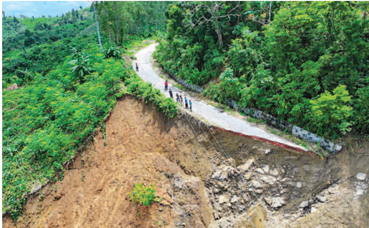
This part of Bandarban-Thanchi road collapsed after a recent landslide due to torrential rain. Workers of the power department have been working to restore electricity supply to the area. The road communications between Bandarban and Thanchi remains snapped. The photo was taken in Parilpar area of Thanchi on Friday.
