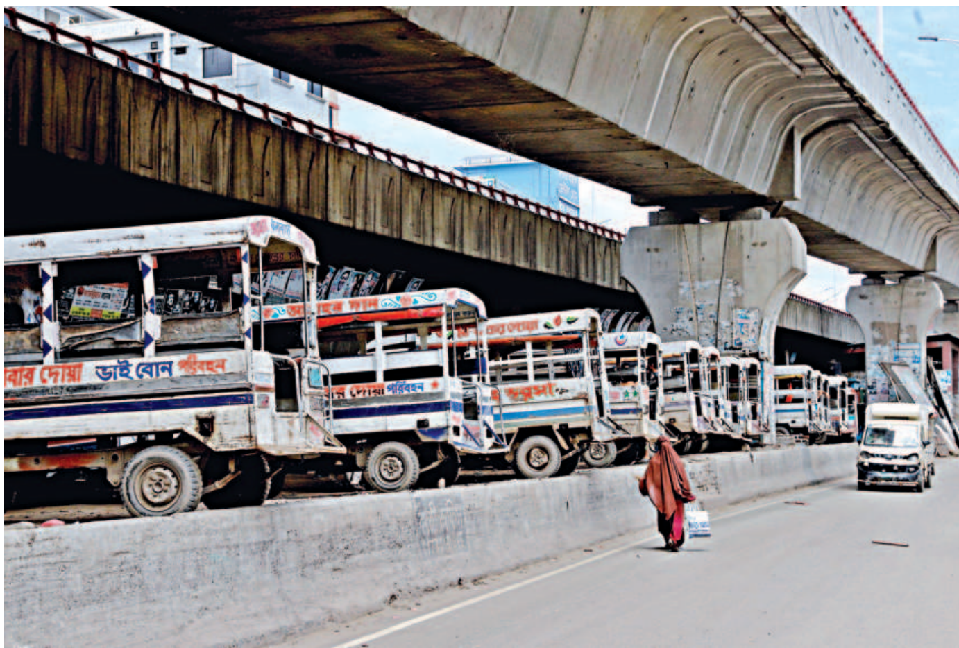
Human haulier companies have illegally turned the space under Mayor Mohammad Hanif Flyover in the capital's Jatrabari area into a parking lot. The photo was taken recently.
