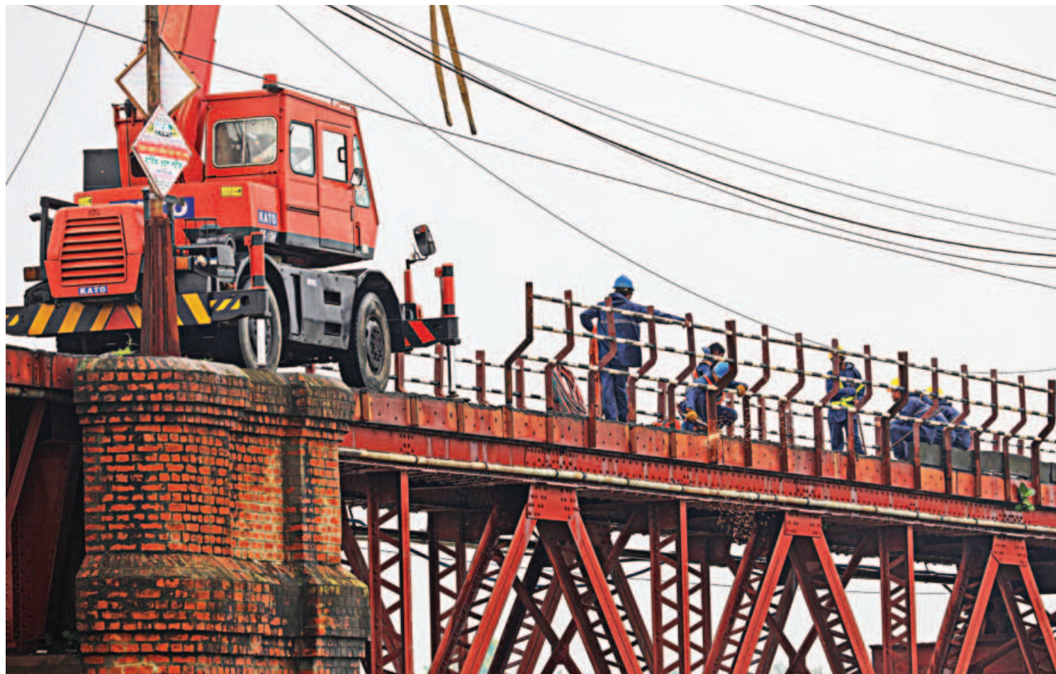
Workers renovating the Kalurghat bridge over the Karnaphuli in Chattogram. Traffic on the bridge has been suspended for the work. The rail bridge was built in the 1930s and later it was turned into a rail-slash-road bridge. This bridge is key to the Dhaka-Cox's Bazar rail service schedule to start this year.
