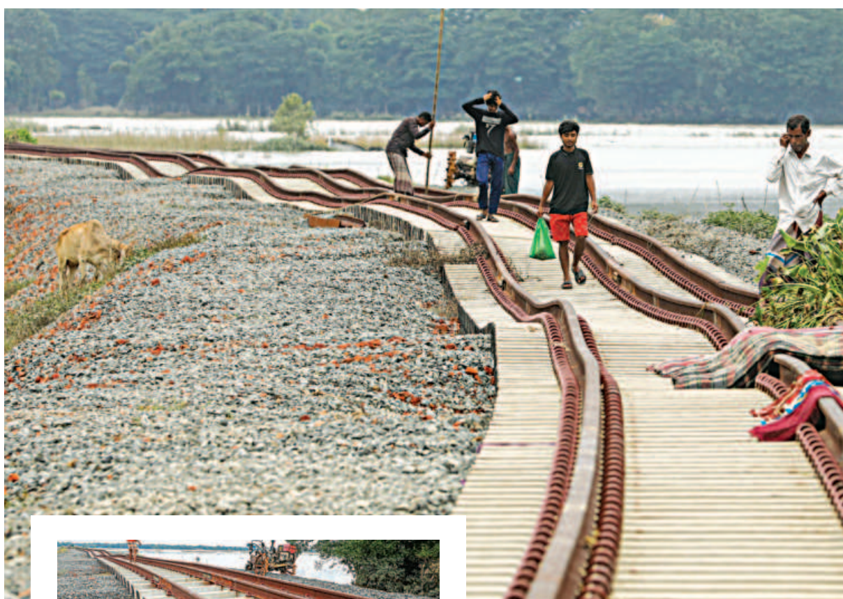
Even before its inauguration, the Chattogram-Cox's Bazar rail line has been badly damaged by floods in Keuchia of Chattogram's Satkania upazila. A vast swath of the upzaila went under water last week. The photos were taken on Sunday.
