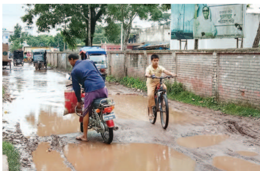
A portion of Kendua-Netrakona Road has remained dilapidated for long, but the authorities have turned a blind eye to the woes of its users. PHOTO: COLLECTED
