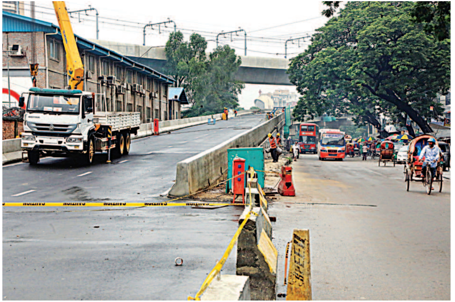
The Airport-Farmgate section of the Dhaka Elevated Expressway is nearing completion in order to be ready for the September inauguration. The photo taken yesterday in Farmgate shows the expressway's exit ramp at Indira Road. PHOTO: PRABIR DAS
