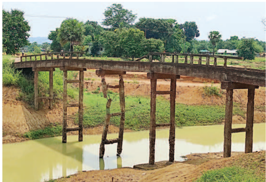
This old bridge at Promod Karbari Para in Rangamati's Baghaichhari upazila has remained in a vulnerable condition, posing threat to a fatal accident. PHOTO: STAR
