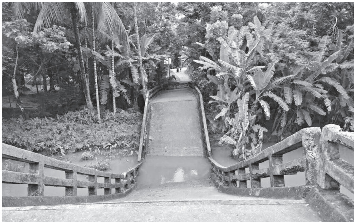
More than 100 bridges constructed over various canals in Barguna remain dilapidated due to a lack of maintenance. As a result, locals, especially workers and students, continue to suffer.
