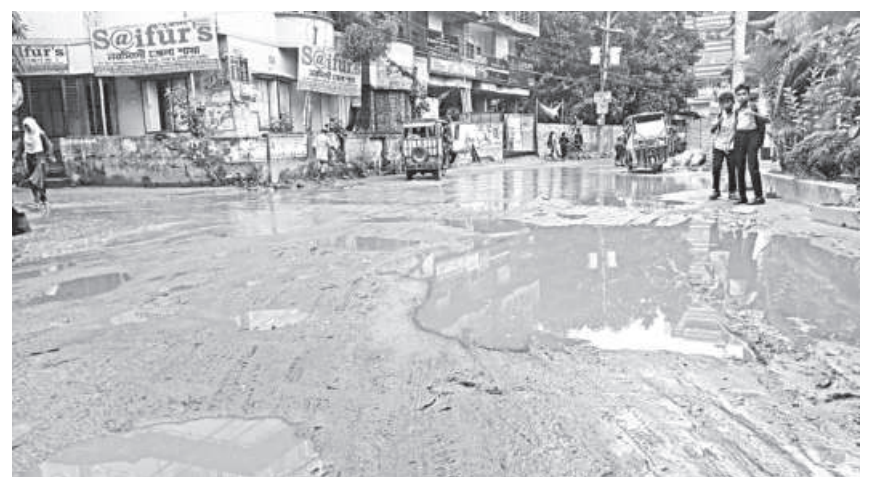
Over 100 ditches and potholes have developed on the roads in Narsingdi town that pose a risk of accidents. The situation gets worse during the monsoon when rainwater accumulates in those craters.
