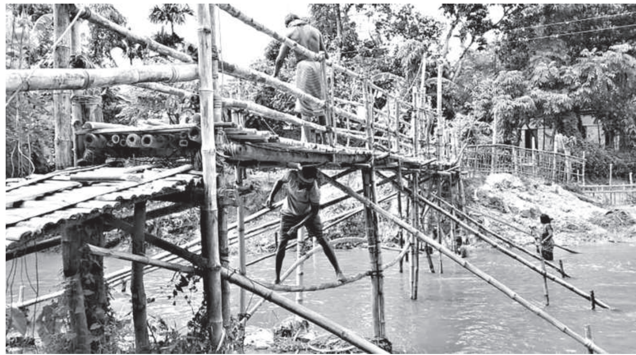
Alor Dishari, a student-led organisation, constructed this makeshift bridge on Bilashchhora canal to ensure commuting for hundreds of students in Dhobighat area of Sreemangal's Kalighat union.
