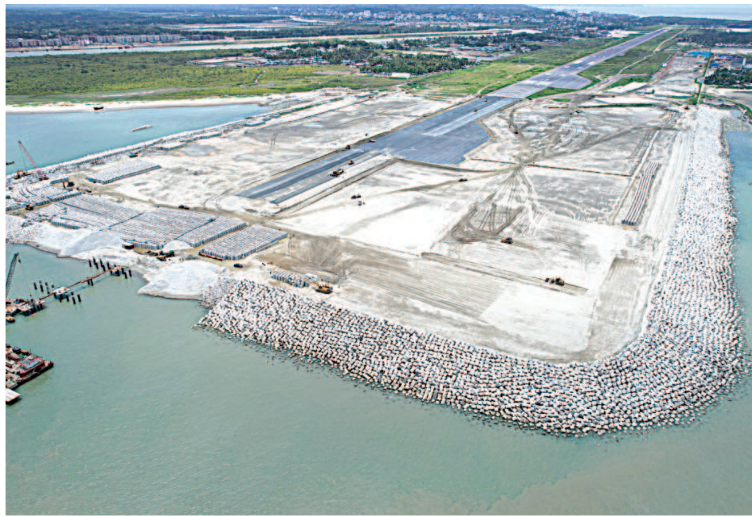
An aerial shot of the expansion work on Cox's Bazar Airport's runway that runs into the sea. It is expected to open by December this year. The photo was taken recently.
