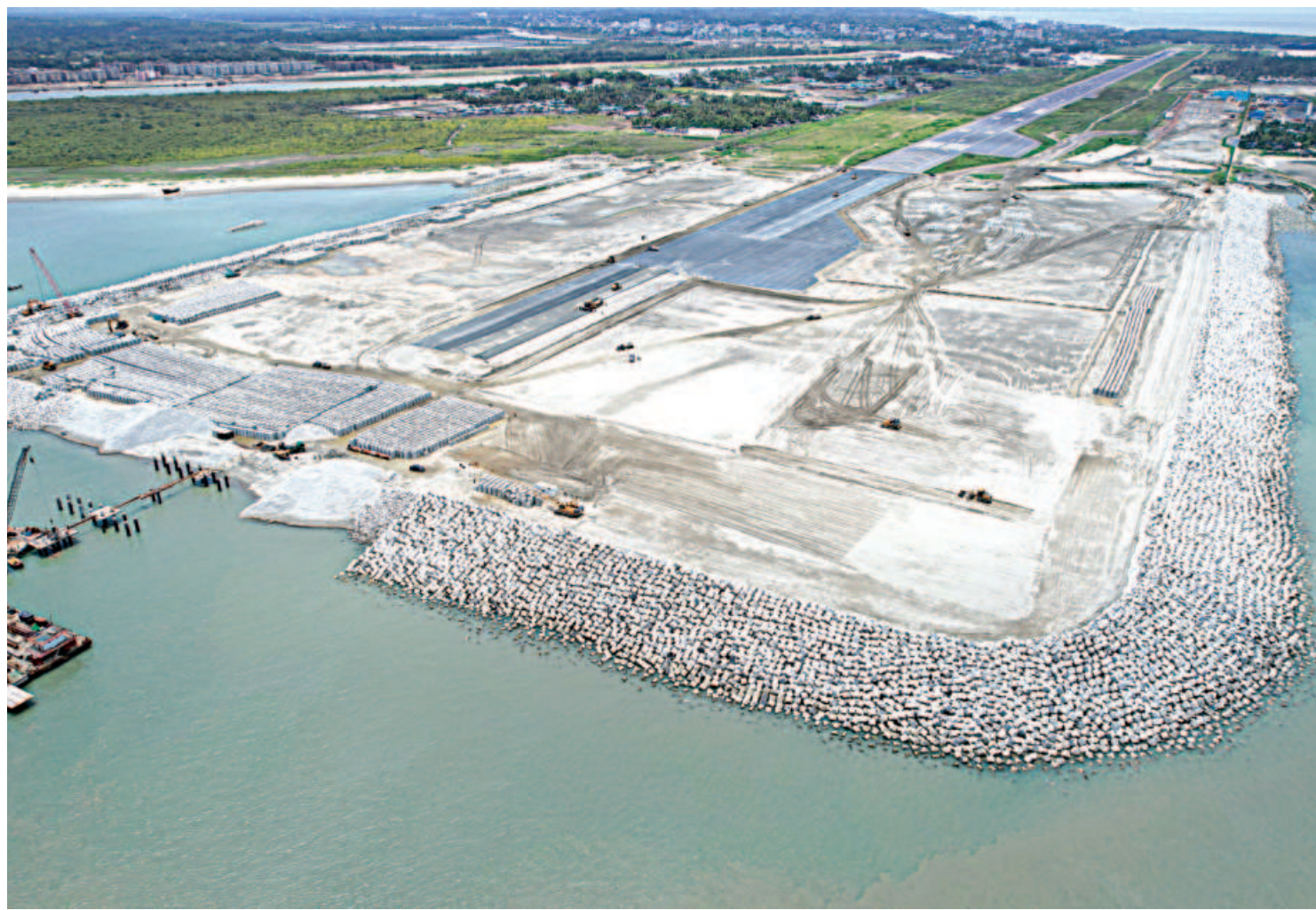
An aerial shot of the expansion work on Cox's Bazar Airport's runway that runs into the sea. It is expected to open by December this year. The photo was taken recently.
