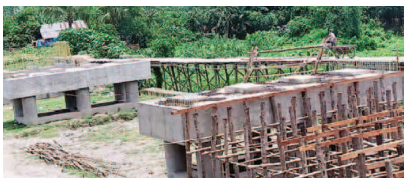
One of the two under-construction bridges over the Betna river on Gorpara road in Jashore's Sharsha upazila.
