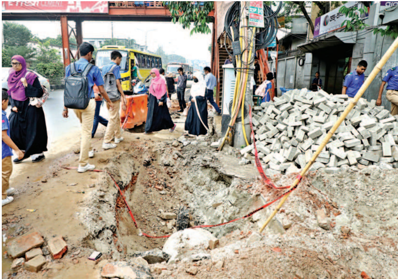
Pedestrians, especially school-goers, are facing difficulties crossing the Jahangir Gate area as construction materials for installing sewerage pipes have been left on the pavement. The photo was taken yesterday.
