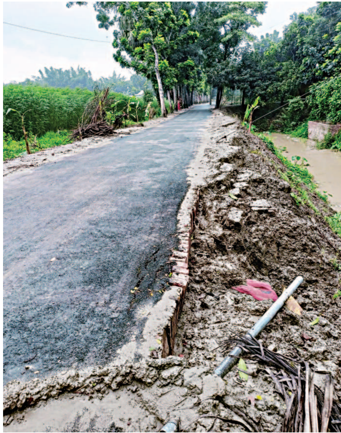
Part of this road in Faridpur Sadar upazila has collapsed just a week of its construction.
