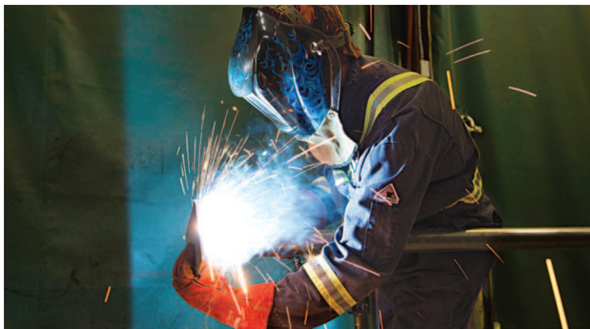
A welder works at a supply and service company in Alberta, Canada.
