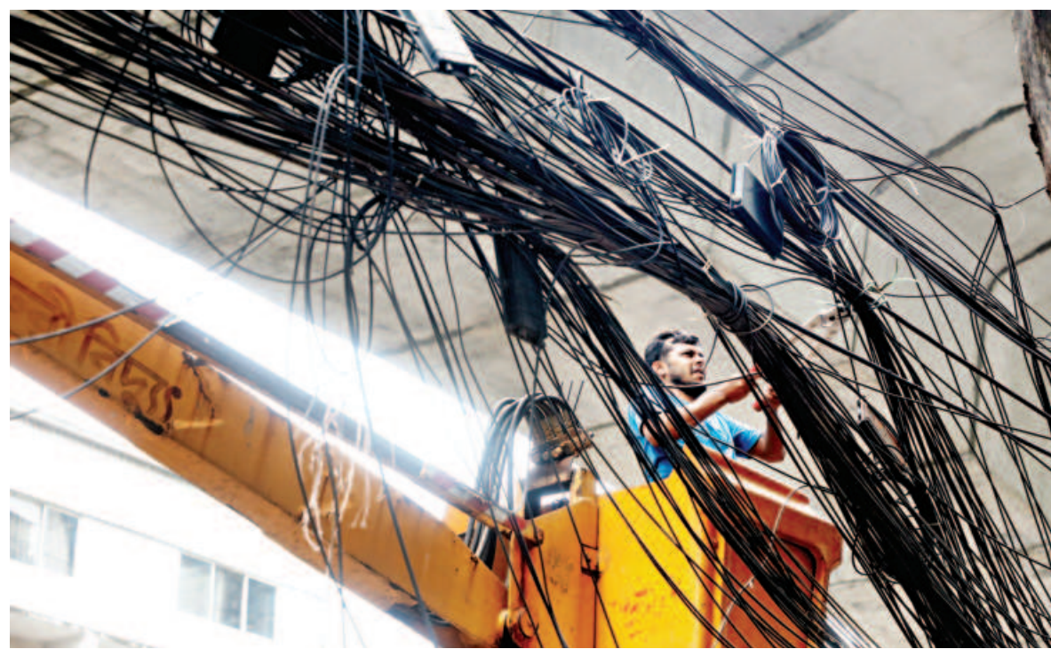
A city corporation worker removing a tangled web of overhead cables, which has been a long-standing nuisance for Dhaka residents. The photo was taken in Paltan area yesterday.
