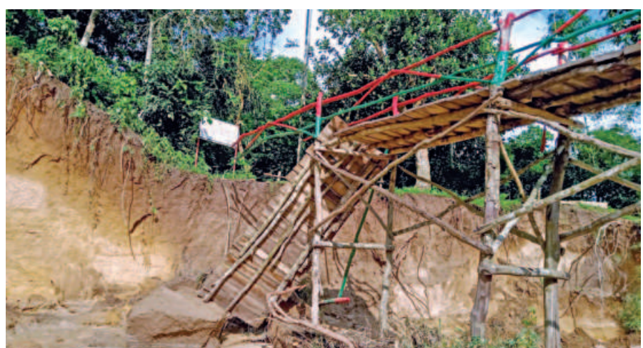
This makeshift bridge over Satchhari Canal in Habiganj’s Chunarughat upazila collapses on Tuesday due to landslide caused by continuous rainfall in the last couple of days.
