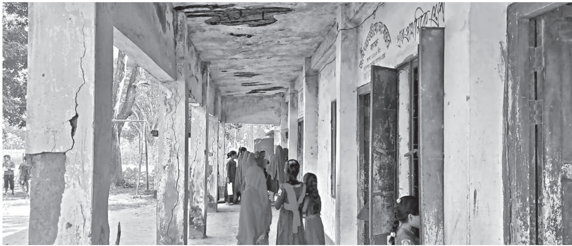
Students of Golgaon Government Primary School in Habiganj's Chunarughat upazila attend classes at the worn-out schoolhouse that has turned risky due to lack of renovation for long.
