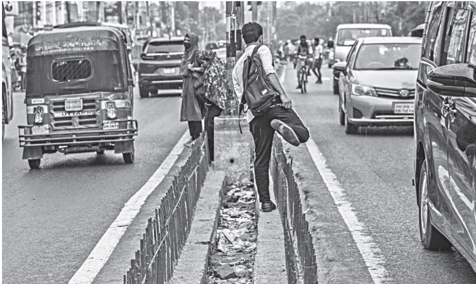
With speeding vehicles coming from both directions and no foot-over bridge nearby, pedestrians have to leap over the iron rods on the under-construction median to cross the capital's Satmasjid Road. This photo was taken yesterday near Jigatola intersection.
