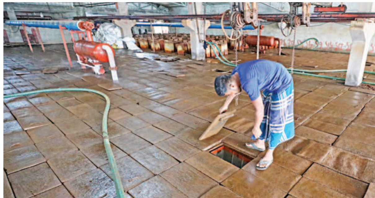
A worker checks on the progress of ice forming inside a metal can at a commercial ice plant in Chattogram. Immersed in a tank of refrigerated sodium chloride brine, the water-filled rectangular cans usually take around 18 hours to form blocks of ice. However, nowadays it is taking around 36 hours due to the frequent power cuts the country is having to deal with over the last two weeks. This has led to a drop in the daily production of ice blocks at this factory from 2,313 to just 500 to 600. The photo was taken at Fishery Ghat last Thursday.
