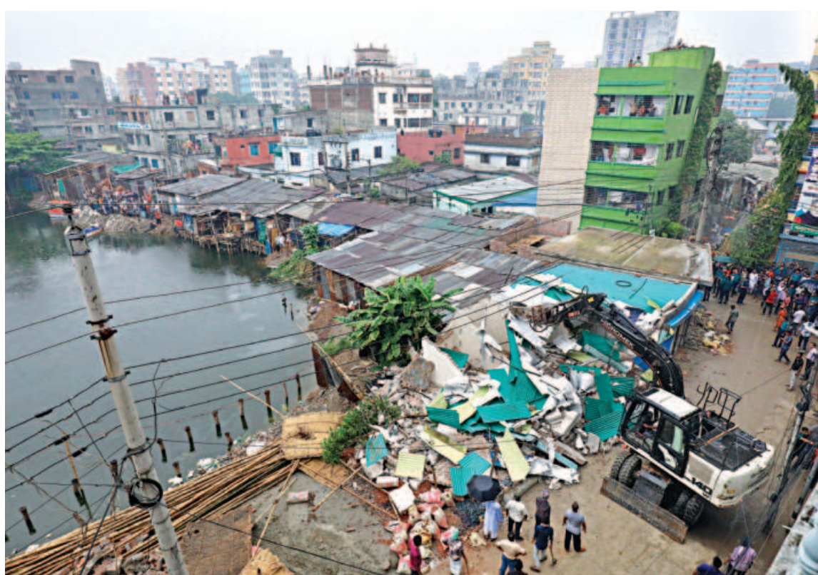
An excavator demolishing an illegal structure on the bank of DIT pond at Gendaria in the capital yesterday. Rajuk, in a drive, knocked down around 100 such structures to free the waterbody.
