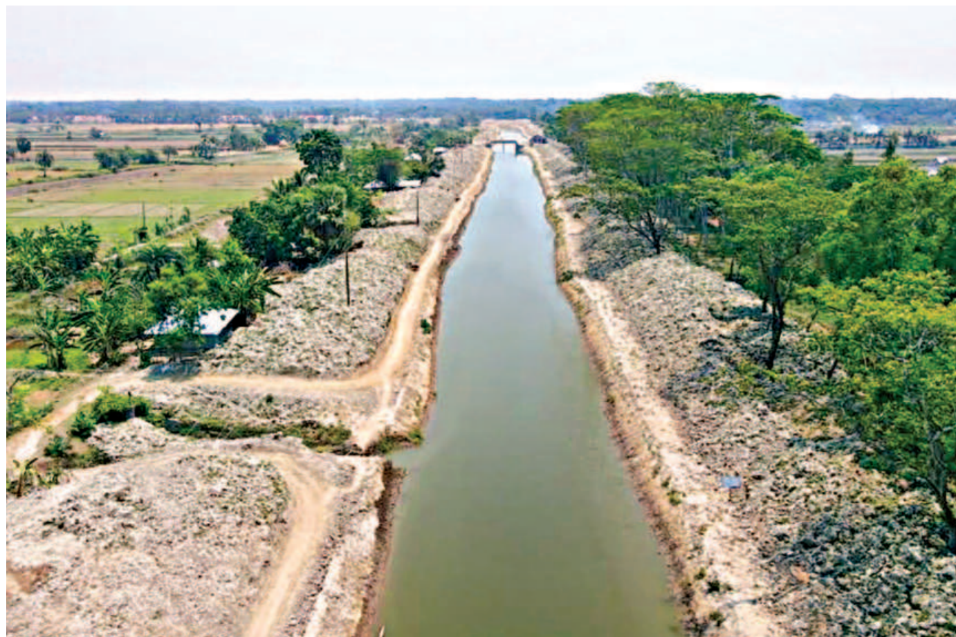
A re-excavated canal, known as Mora Posur, gets a new lease of life. Seven such canals, including this one, were re-excavated in Betaga union of Bagerhat's Fakirhat. Now farmers are getting irrigation water from them. The photo was taken in Betaga village recently.
