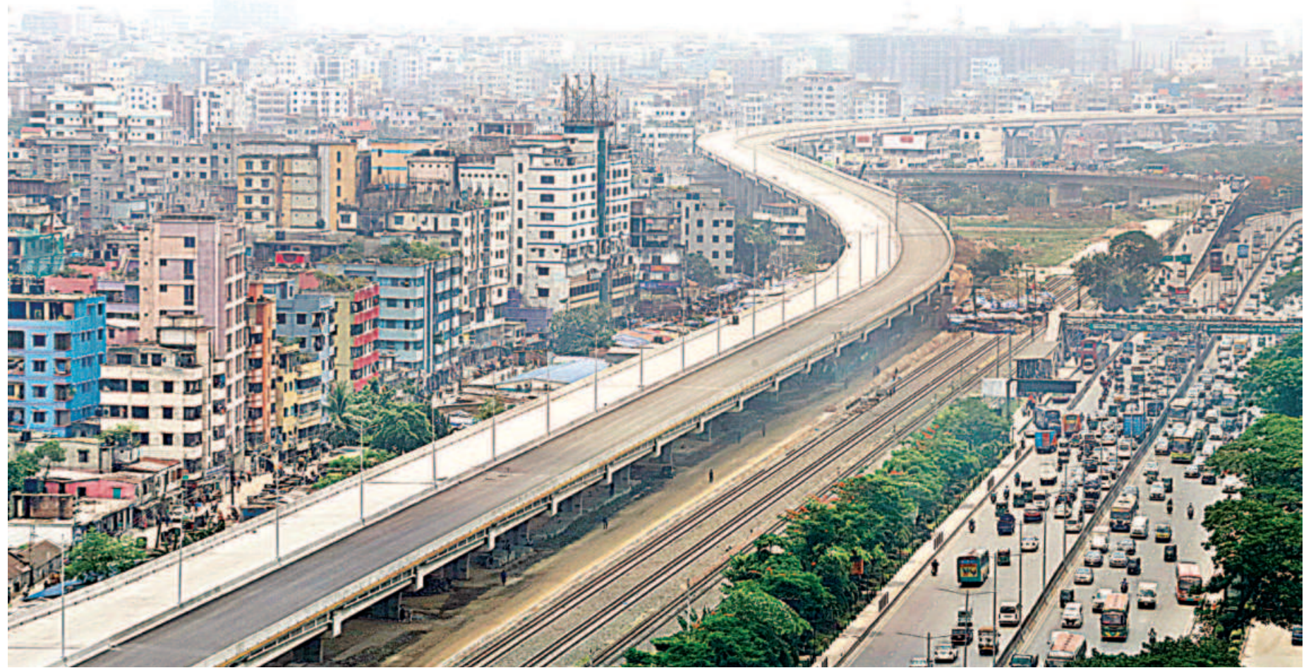
A partial view of the under-construction Dhaka Elevated Expressway. The project has made a major progress as the authorities have already asphalted one of the two lanes of the expressway in the capital's Khilkhet area. After changing the project deadline for several times, the authorities now want to open a section, stretching from the airport to Tejgaon, to traffic by November this year. The photo was taken recently.
