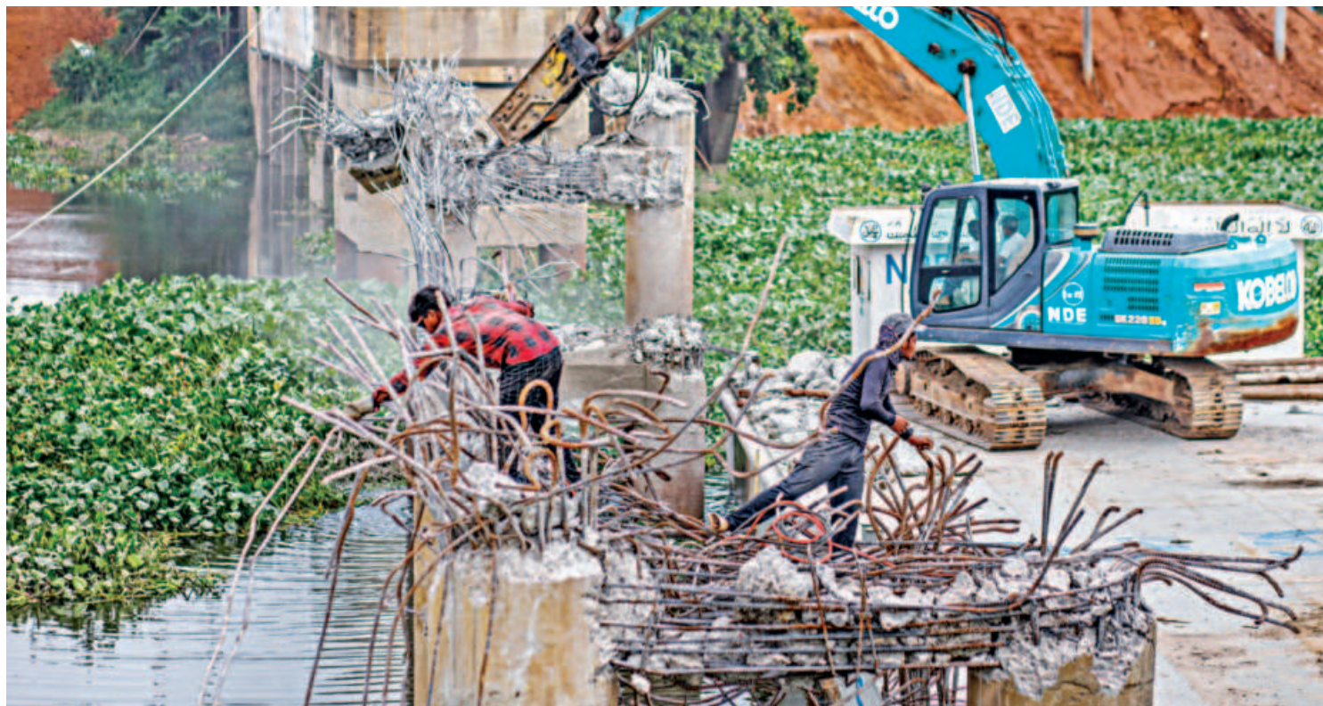
Amid rods protruding precariously and no safety harnesses in sight, workers continue demolition work of a bridge in the Magrakanda area of Savar-Keraniganj road yesterday.
