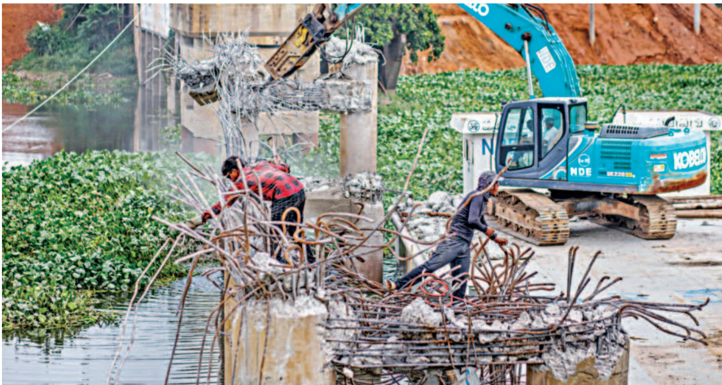
Amid rods protruding precariously and no safety harnesses in sight, workers continue demolition work of a bridge in the Magrakanda area of Savar-Keraniganj road yesterday.
