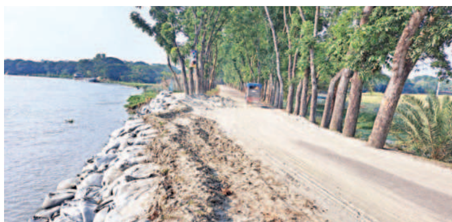
Erosion by the Ramnabad river has devoured a large portion of this flood control dyke at Tetultala village in Patuakhali's Galachipa upazila, threatening collapse of the dyke any moment.
